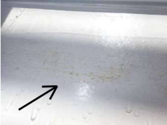
Photo 25-1 Close up of window sill staining.
